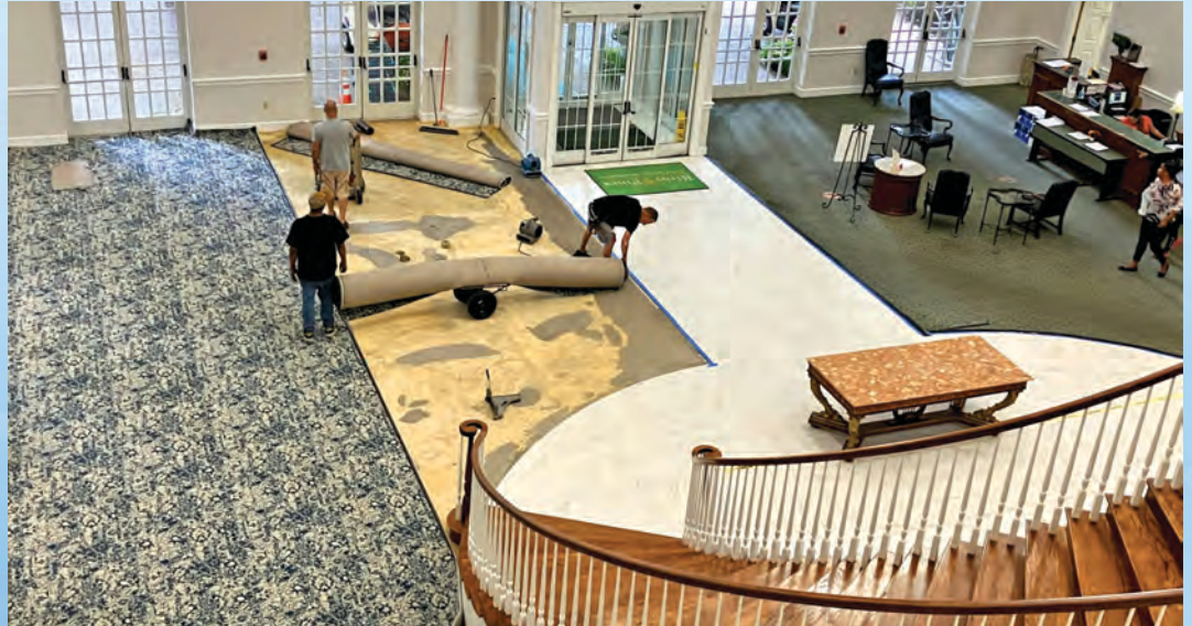
As the Lobby renovation continues, the new carpet is being installed. Photo by Sylvia Statham
